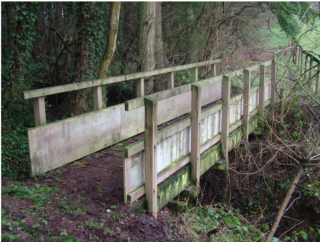
Bridleway Bridge. The sheet boarding for the kick boards should be replaced by lower rails
