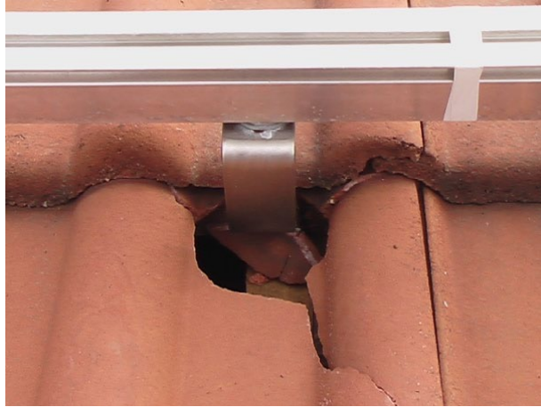
Figure 7 A roof tile damaged by roof hooks for attachment of PV modules (source: VdS 3145)
