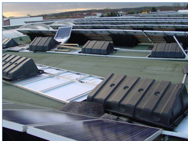
Figure 4 Example of storm damaged PV modules on the roof (source: VdS 3145)
