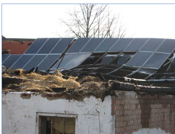
Figure 6 Fire damaged roof with destroyed PV modules (source: VKB)
