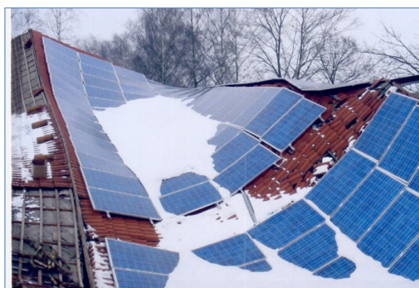
Figure 5 A roof with PV modules collapsed under snow load (source: VdS 3145)
