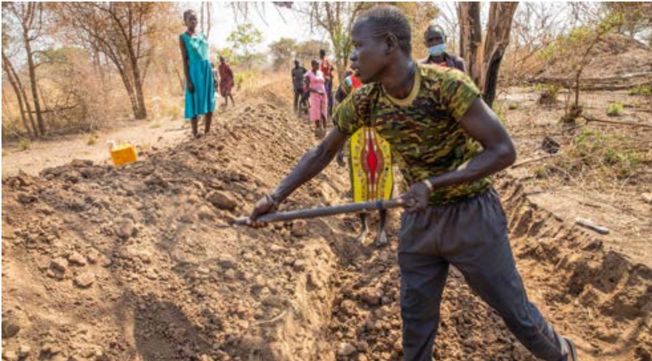
A man from among-Piny digging the channel to create a dyke that will prevent water to enter the village during cash for work project to support the community from flood in Rumbek on Friday, March 12, 2021. Photo: FAO/Mayak Akuot
