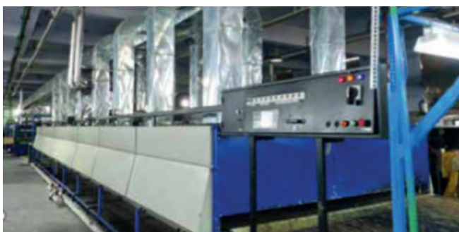
Distribution hot air into drying tunnels
