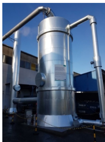
Figure 2. Working CTBB during tests of bio-purification of air in real conditions of Enduser. Source: own elaboration
