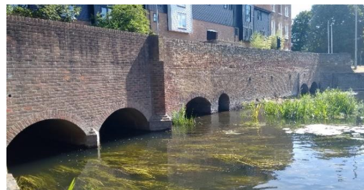
Figure 2. Barrier 1 to Fish Passage at West Drayton Mill
